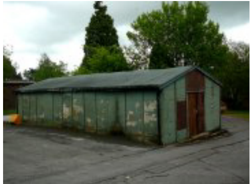
(Right) A dilapidated building
