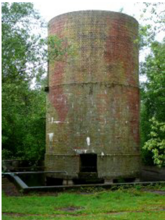
(Right) Cooling Tower
